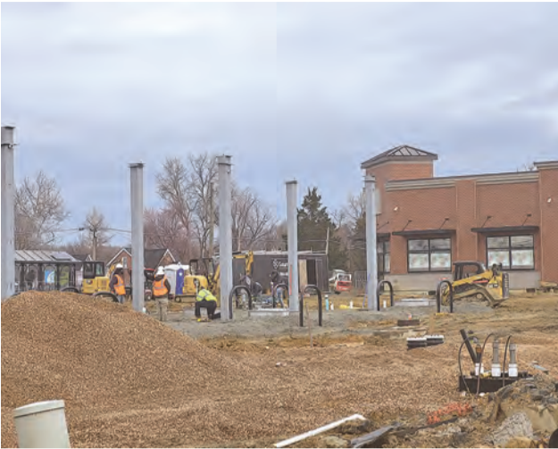
In the 8620 Richmond Highway, a new 7-11 takes shape to give shoppers in that part quick-shop option.
