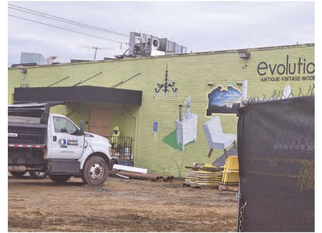
The Revolution consignment store in Penn Daw is going down and will be replaced by townhouses and another building.
